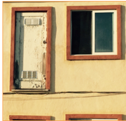
2nd story door, missing stairs
